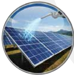
SOLAR PLATE WASHING
